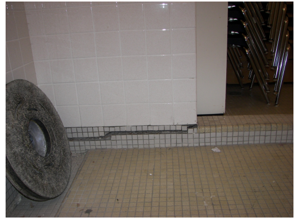
(1978) (Boys Locker/Shower 17) - concrete slab on grade has settled.
