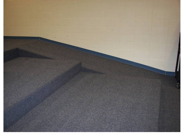
(1978) (Music 8) - wood ramp is too steep.
