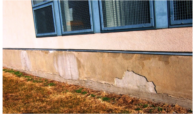
Damaged acrylic stucco finish.
