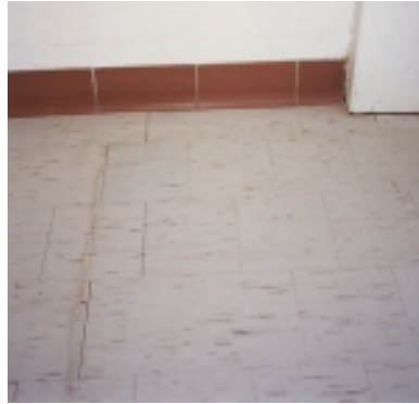
Typical Corridor Floor Heaving, 1960 Corridors
