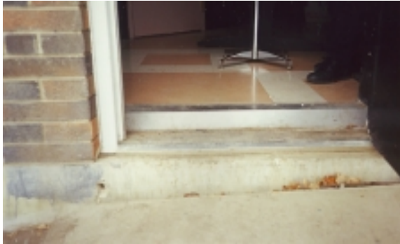
Settlement Outside South Façade, 1962 Portion
