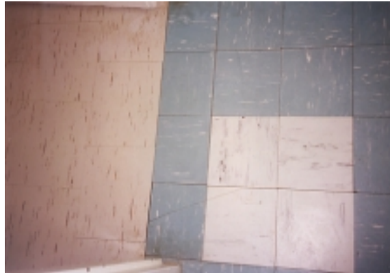
Loose Asbestos Tiles at 1960 Classrooms
