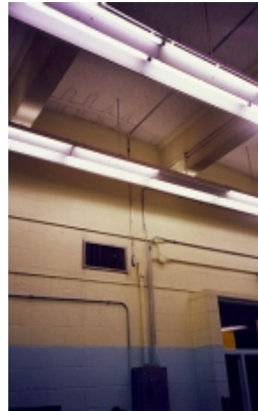
Roof Leak Above Electrical Panel, Room 153
