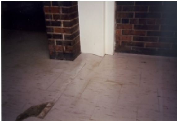
Floor heaving at 1960 Structure
