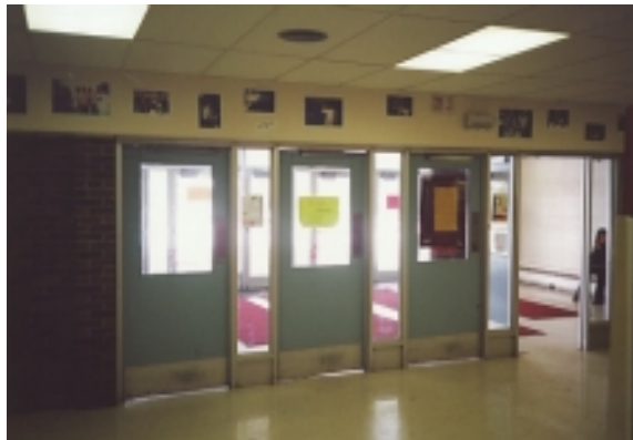
Compressed Door Frame at East Entrance
