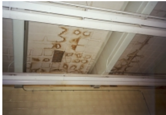
Roof Leaking at South Wall of Industrial Arts
