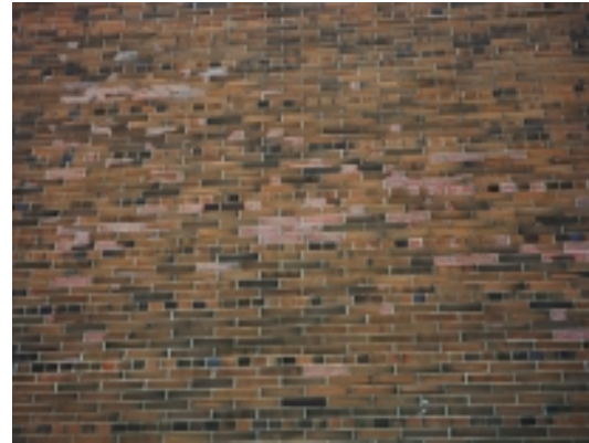
Efflorescence/Spalling at North Walls
