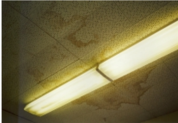
Roof Leakage at Classrooms - 1960 Wing
