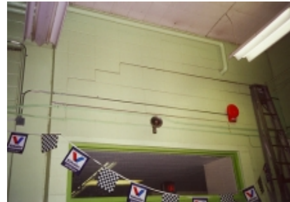
Wall Cracking at Automotives
