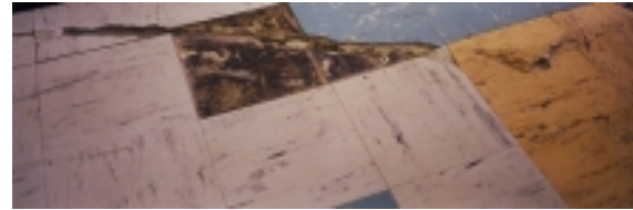
Floor Displacement at Room 204
