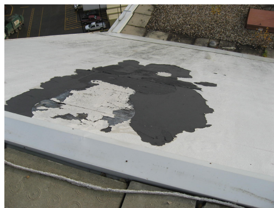
Deteriorated elastomeric coating on sloped roof section A3.
