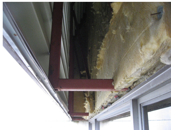
Missing metal soffits above windows.
