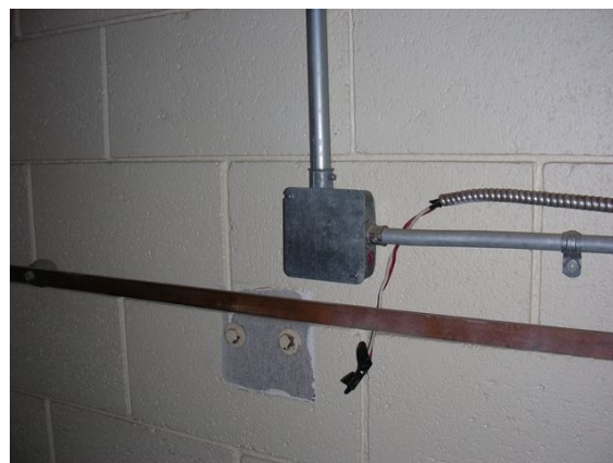
Wiring in medical gas storage area is not rated for explosion proof area.
