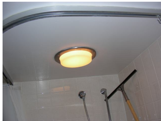
Incandescent lighting in showers is not energy efficient.
