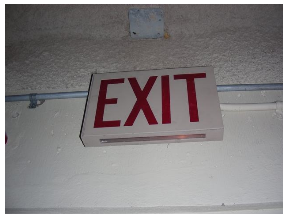
Incandescent exit sign is inefficient and has a short lamp life.
