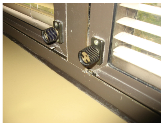
Removable inner pane with damaged rubber gasket throughout the majority of the window units.
