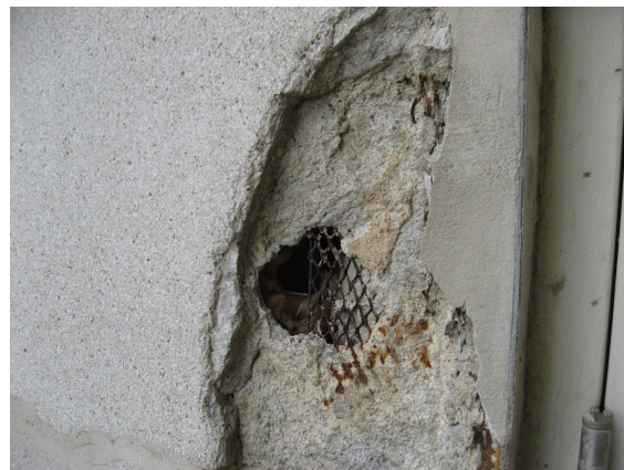
Missing finish coat on exterior wall assembly observed in several locations. Smoke test was conducted in this area.
