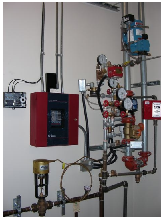
MRI Pre-action system is not tied into fire alarm system.
