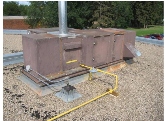
Rooftop unit serving Cafeteria.
