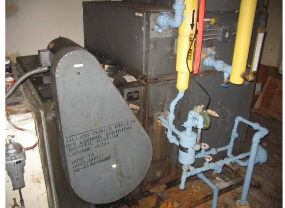
Multizone unit AS-8 serving 1966 section.
