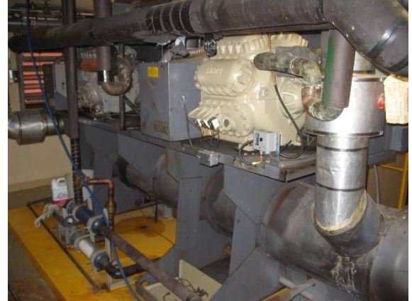
Chiller located in Mechanical Room.
