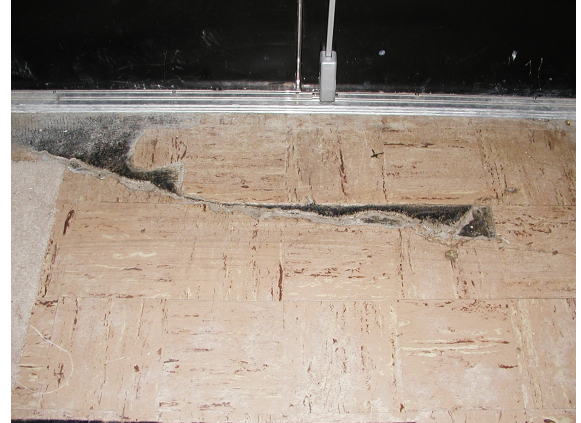
Failed VAT flooring at emergency exit, due in part to shifted gym floor slab.
