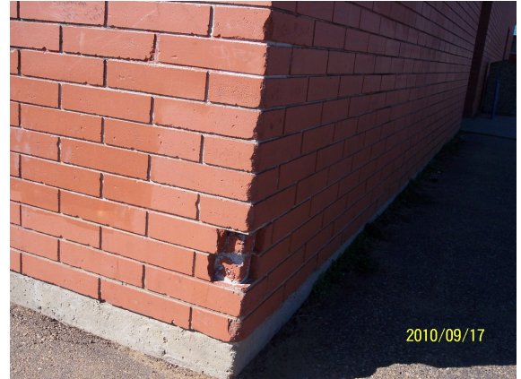
(1973) Addition (Northeast corner) - has damaged giant modular unit bricks.
