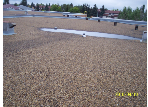
(1989) Original Building - has ponding.
