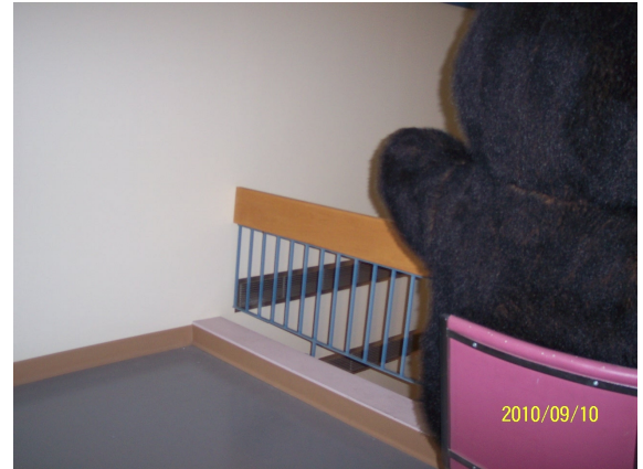
(1989) Original Building (Mezzanine 205) - railing and balustrades are too low and do not meet building code.
