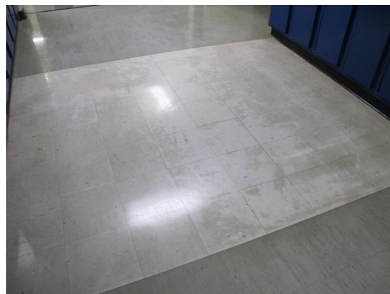
Deteriorated finish on vinyl floor tiles in corridors.
