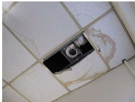
Stained ceiling tiles in the stairwell washroom in the original 1963 Section.
