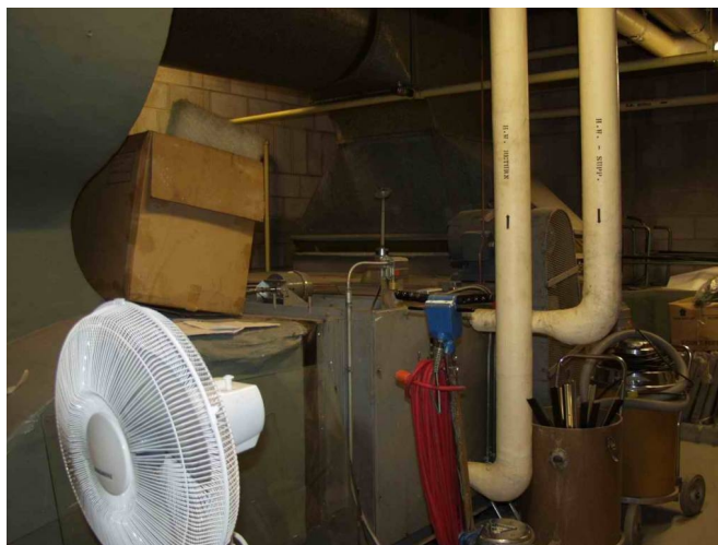
West Wing Air handling Unit. Serves Basement and Main Floor
