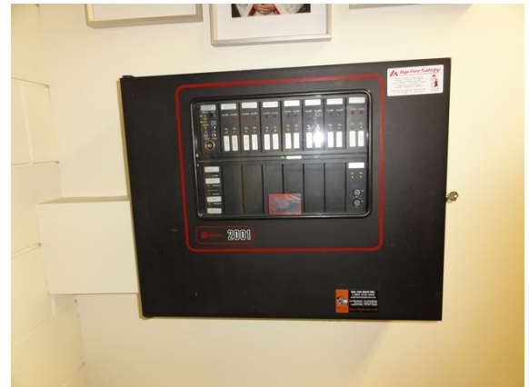
Simplex 2100 fire alarm control panel located in administration area.
