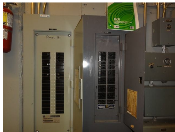
Original Square D (1963) and Westinghouse (1972) branch circuit panels.
