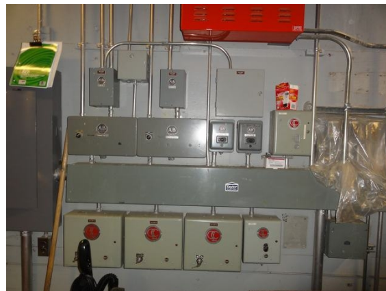
Allen Bradley and CCL motor starters in mechanical room.
