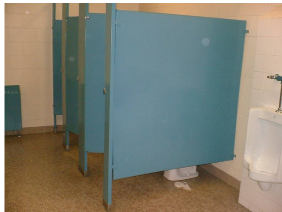
Metal toilet partitions.
