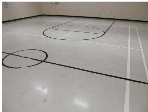
A severe bow throughout the small gym floor in the 1972 Section.
