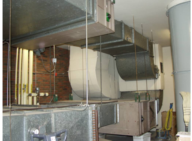
West Wing Air Handling Unit. Serves Upper Floor
