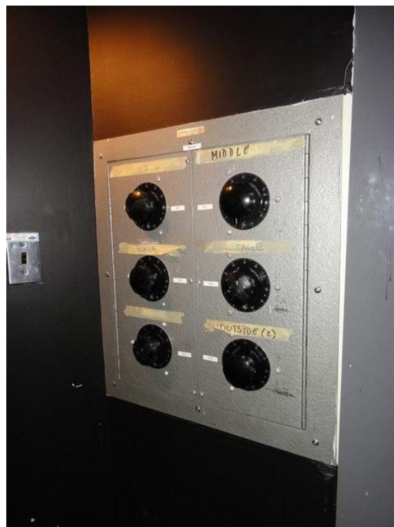
Obsolete dimmer panel on stage.
