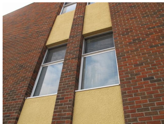
Deteriorated sealant around window assembly.
