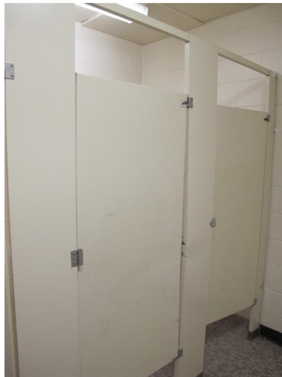
Damaged door panels in washrooms
