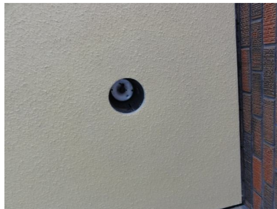
Inefficient exterior incandescent lighting fixture.
