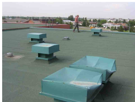
Dented roof caps.
