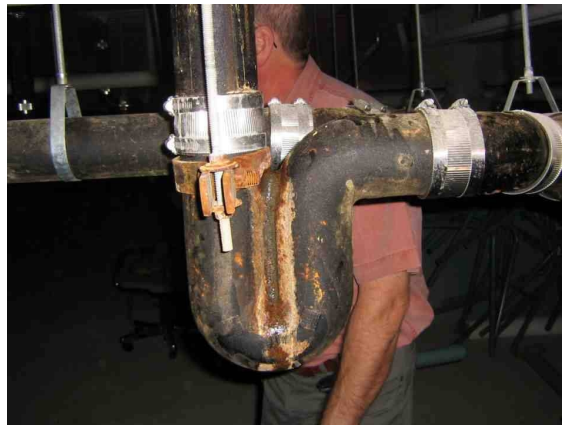
Trap leaking in crawl space.
