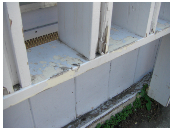
(1968) Circular Building - Classroom Windows have rotten wood sunscreens.
