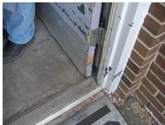
(1968) West Wing (Outdoor Gymnasium Storage) - wood door and hardware are worn out.
