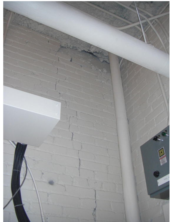
(1930) Original Building (ELEC 029) - load bearing brick masonry walls have cracks.
