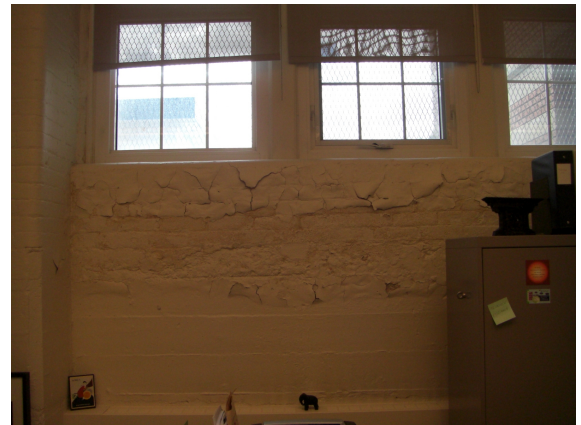
(1930) Original Building (Office 034) - paint has peeled off.
