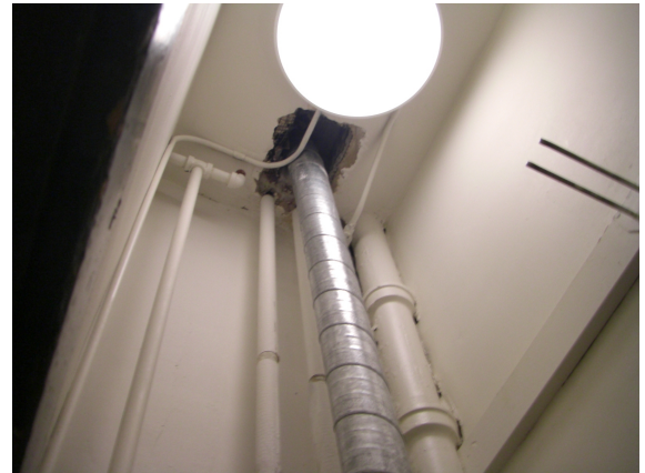
(1930 Original Building (Jan 131) has holes in ceiling.
