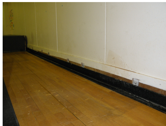
(1971) Addition (Main Floor - Gymnasium 122) - concrete slab has dropped more than 50mm.
