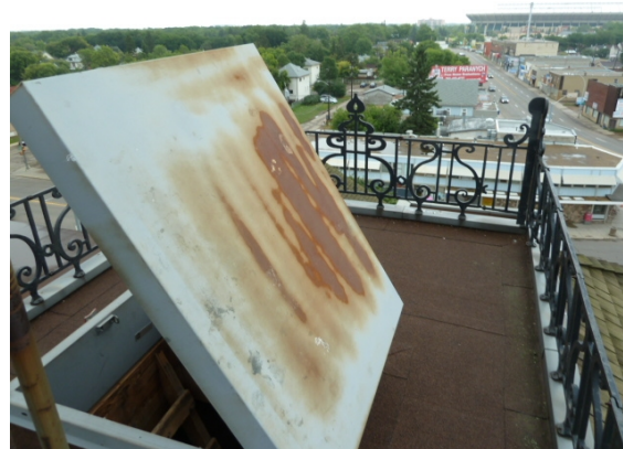
(1908) Original Building (Third Floor - Attic to Roof) - has a rusty metal roof hatch
