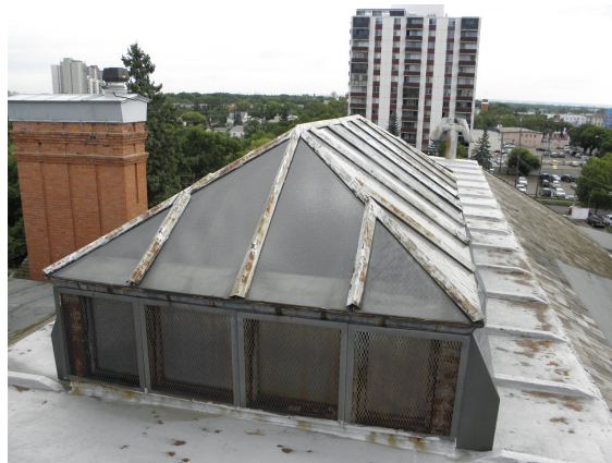
(1907) Original Building - metal framed skylight is rusty.
