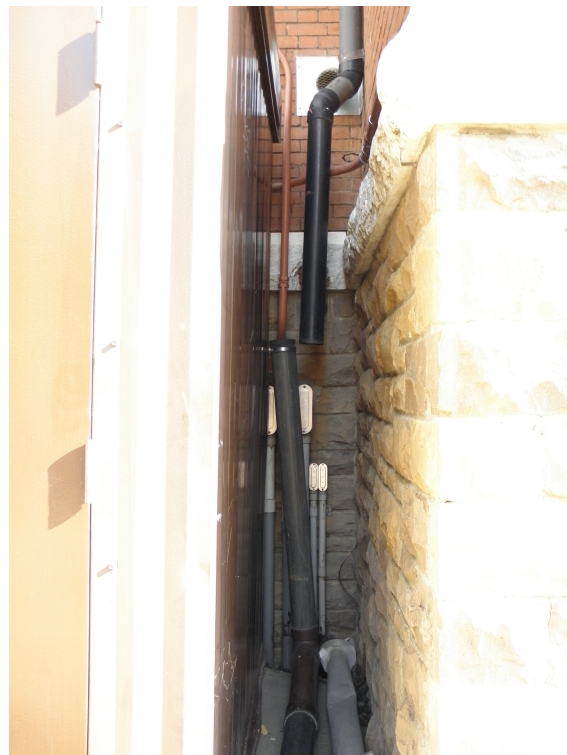
(1907) Original Building (South Wall near Mechanical Room 6) - has damaged downspout. (1 downspout)
