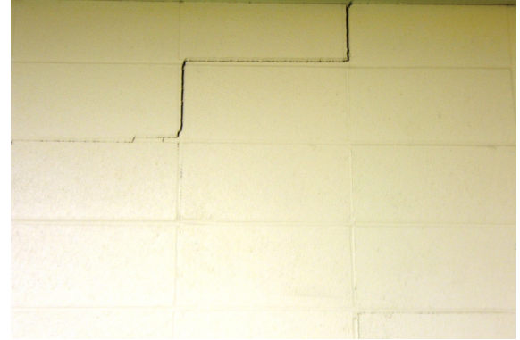
Located in exterior wall of west wing classrooms. Adjacent washrooms present similar condition.
