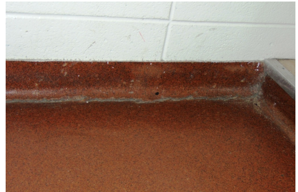
Separation crack located in changes rooms. Similar condition in west side washrooms along exterior wall.
