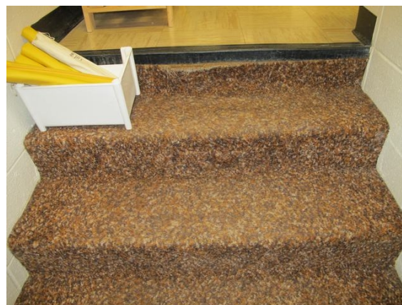
Aged and torn carpet at top of stair.
