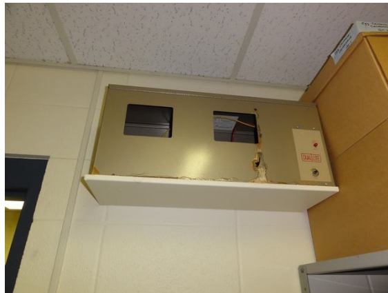
Aged emergency battery unit.
