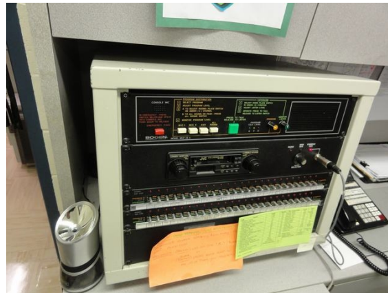
Obsolete Bogen MCP-35A P.A. system.
