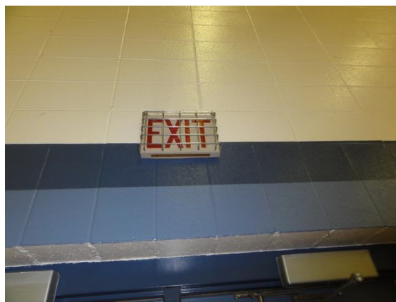
Incandescent exit sign - burned out.
