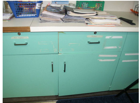
Damaged and mis-aligned doors, peeling plastic laminate.
