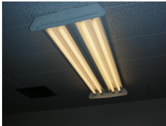
Aged inefficient 4-lamp T12 fluorescent lighting.
