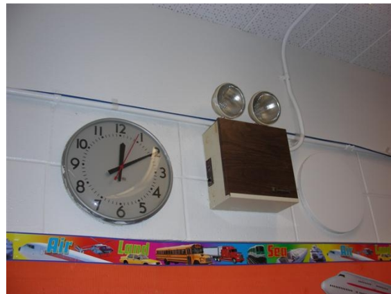
Aged emergency lighting battery unit - not operational.
