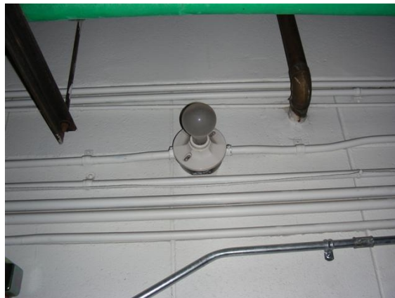
Incandescent emergency lighting fixture.
