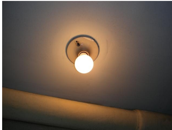
Incandescent lighting in mechanical room.
