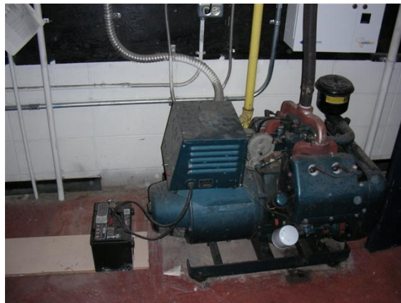
Natural gas emergency generator.
