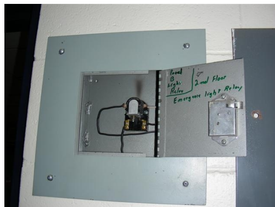
Emergency light relay.
