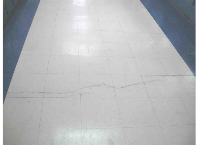
Crack in floor slab near student common area.
