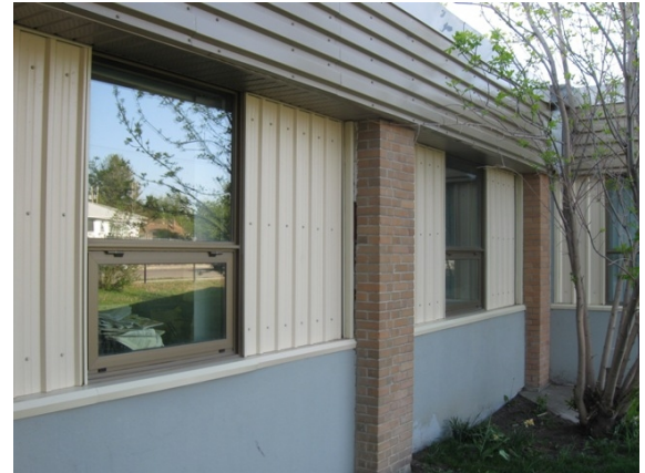
Voids between exterior metal siding and section of brick veneer.
