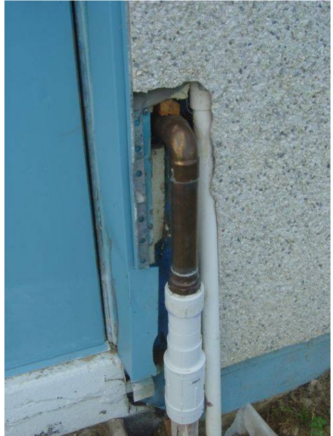
Rock dash stucco needs to be repaired and closed up.
